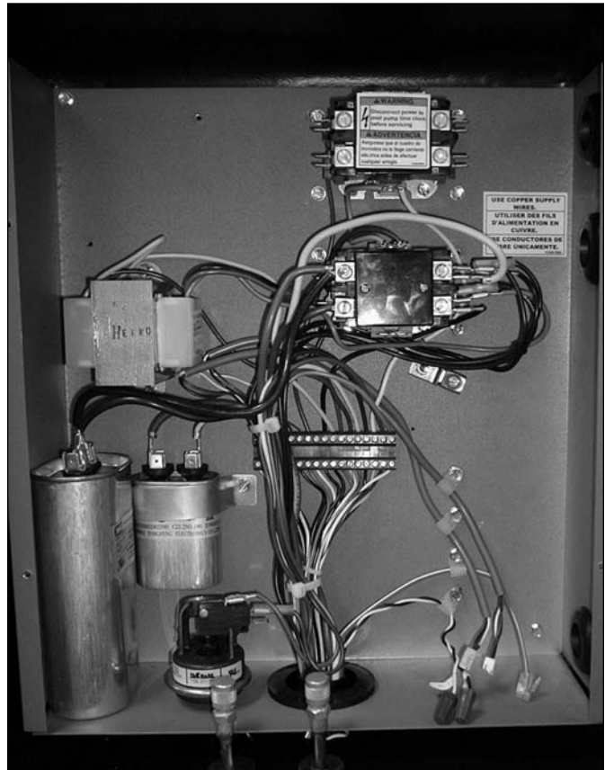
Figure 13. AE-Ti Control Panel, Interior View
